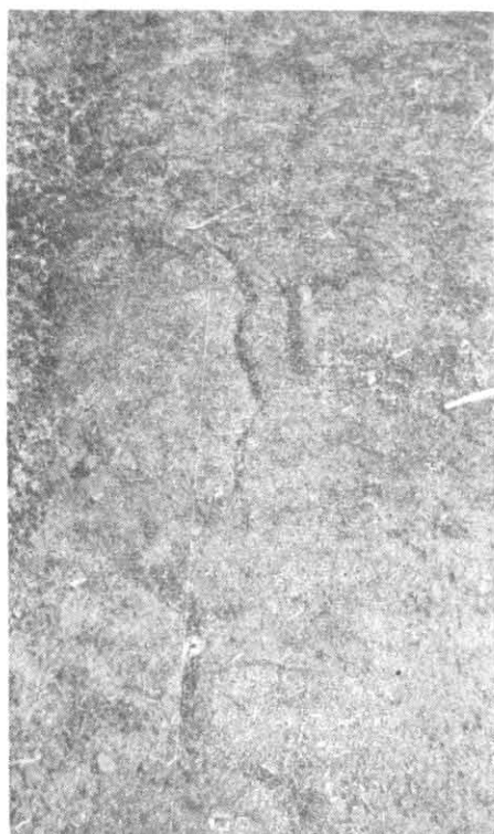
Fig. 8. An irregular shaped crack on the ground near Hirekerur
