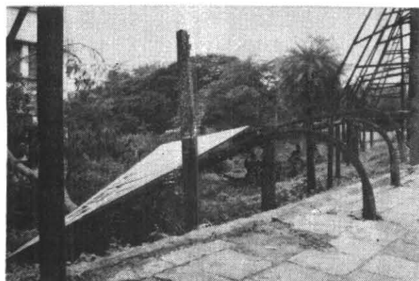
Fig. 3. Guindy bridge, Madras—iron hoardings twisted and bent due to severe cyclonic storm (29-31 October 1994)
