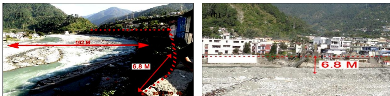
Fig. 13(a&b). Field observation of washed-out areas at (a) Joshiyara market and (b) Joshiyara bridge
