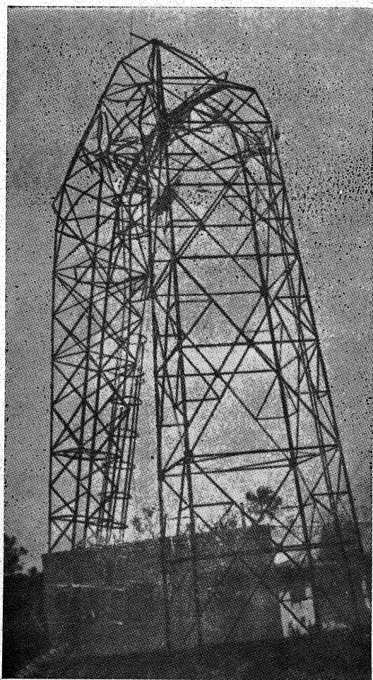
Fig. 9. Aerial mast of wireless repeater station at Man-nargudi damaged by Nagapattinam cyclone
