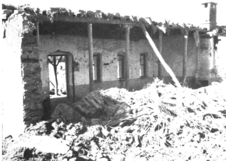
Fig. 3. Police barracks destroyed by rains in Jullundur Cantonment.
