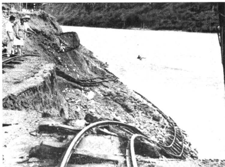
Fig. 1 Railway track of Darjeeling Himalayan Railway damaged due to downpour of rain in June 1950 (Photo : Statesman, Calcutta )
