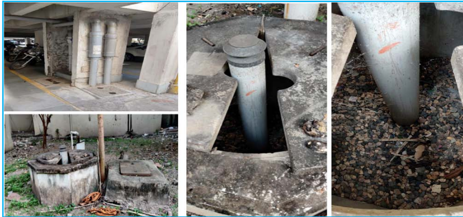
Fig. 16. Rainwater Harvesting system installed in the Residential and Institutional Building
