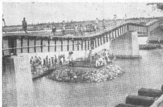
Fig. 3. Chinnaganjam Railway Bridge after May 1969 Andhra Cyclone
