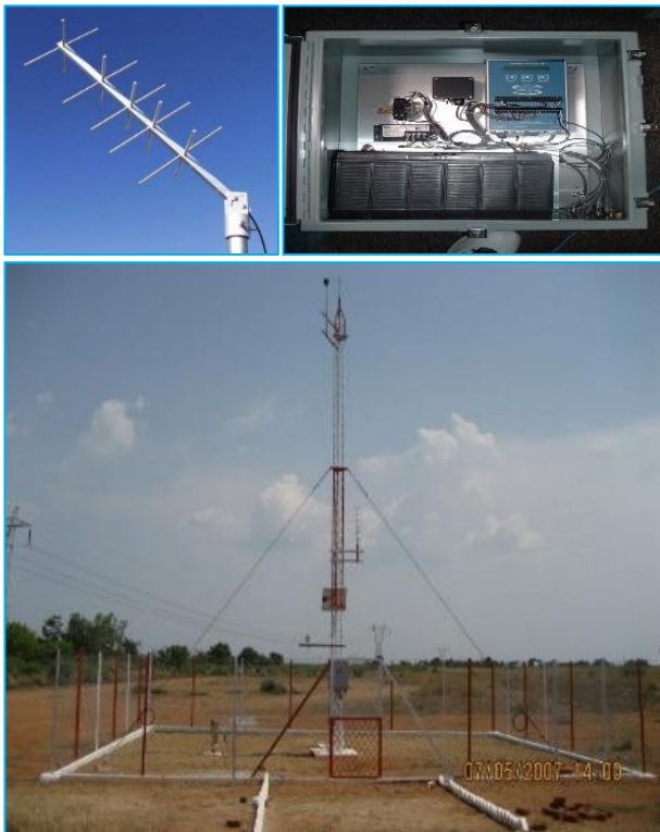
Fig. 37. Typical site installation of AWS
